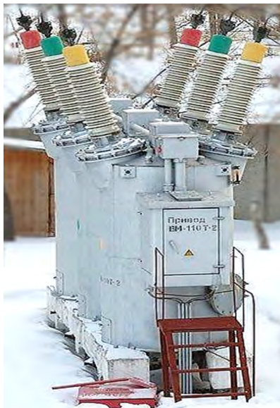
Figure 3.29: Oil circuit breaker MKP-110 (110 kV) on traction substation 110 kV 50 Hz/3.3 kV DC of railway, Toliatti city, Russia. By: Vivan.
