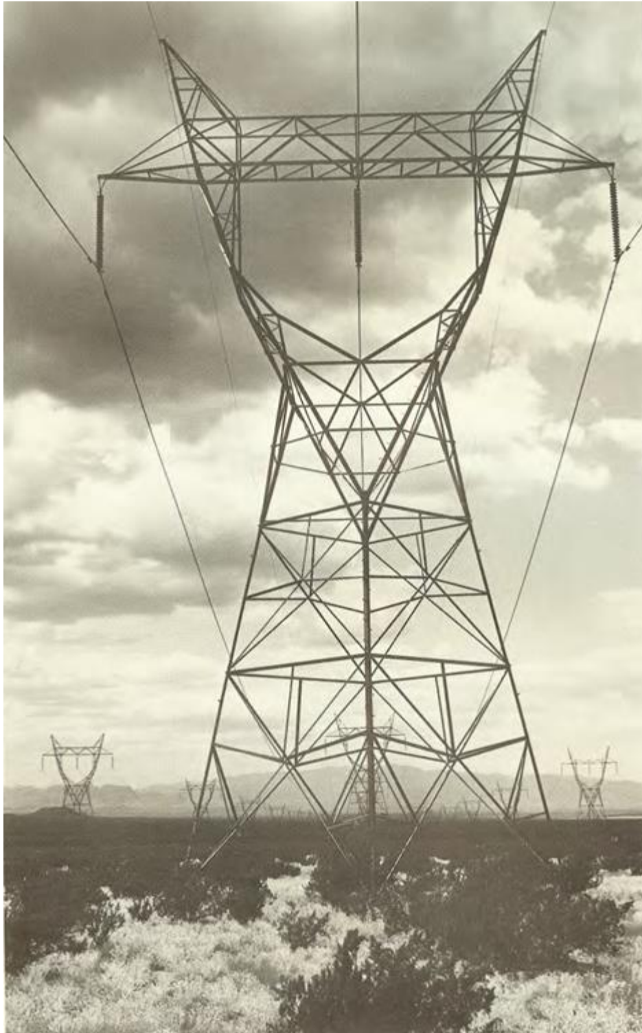
Transmission lines carry Hoover Dam power across the Nevada desert to southern California.
