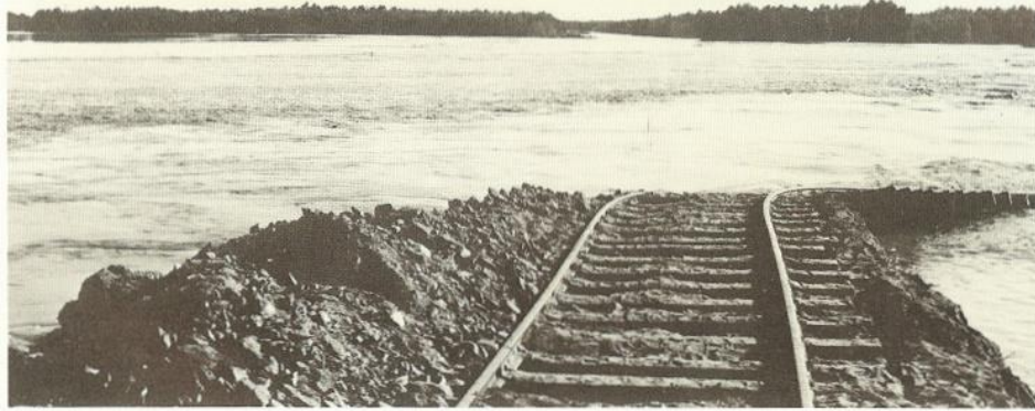
Southern Pacific Railroad tracks in the Imperial Valley were washed out during the 1905-06 flood.
