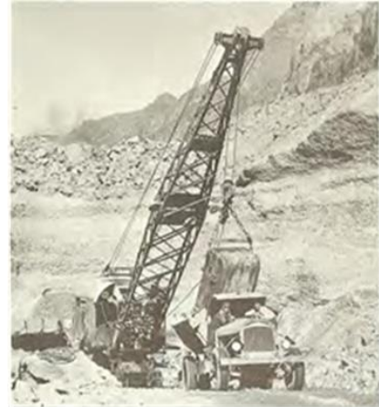
Workmen excavated thousands of tons of riverbed material to reach foundation bedrock for the dam and powerplant.
