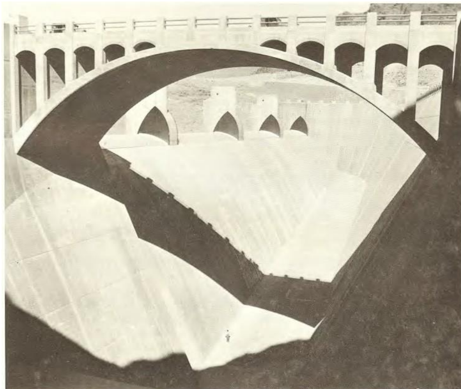
Arizona spillway, 1936. Spillways are 650 feet long, 150 feet wide, and 170 feet deep. Note man at bottom of spillway.
